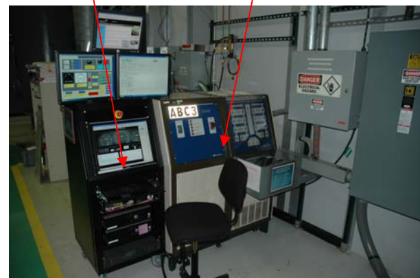
Fig 2(a). Battery HIL control and data acquisition Rack, and high voltage DC power supply
